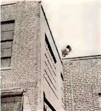
Sound systems are needed in busy industrial plants.
